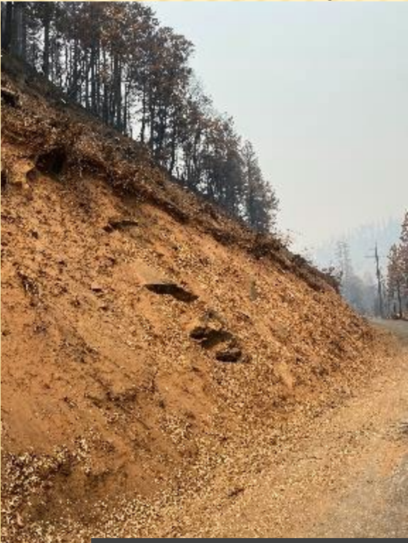
Active landslide along 7F002
